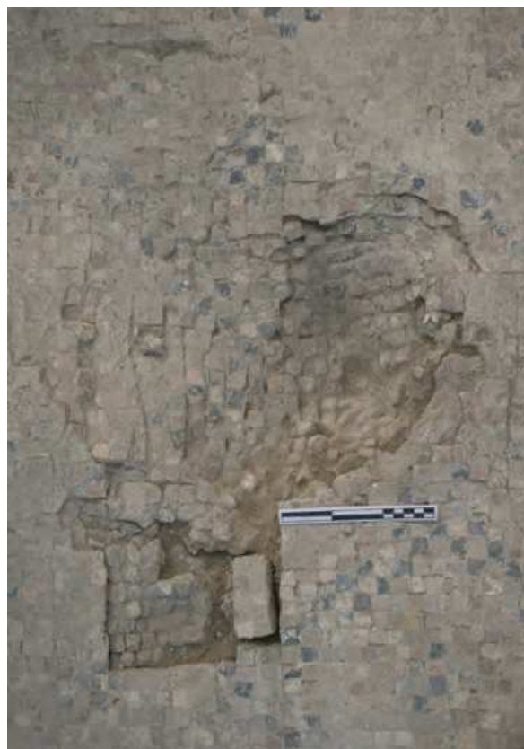
Fig. 6. Serious surface deformation and large lacunae appeared throughout the mosaic carpets as a result of the earthquake of AD 749 (photo: J. Burdajewicz)
