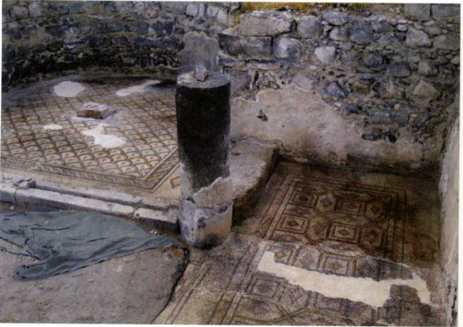
Fig. 4: Once the earlier layers were investigated, a new bedding was prepared and the mosaic was relayed in its original position in the south aisle of the church.
