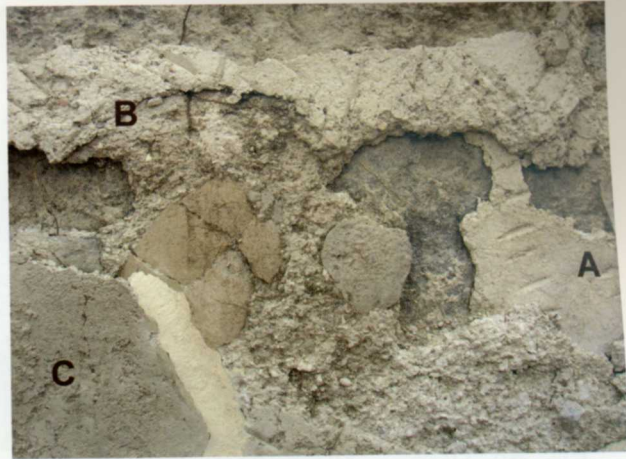
Fig. 80, Hippos, NWC, collection vat of the winery, three layers of hydraulic plaster: [A] the lowermost one of good quality, [B] thick layer containing crushed potsherds, [C] thin external coating. Note hatches on layers [A] and [B]
