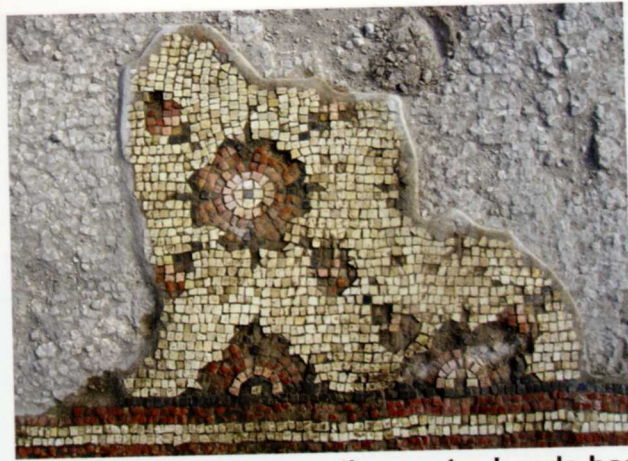
Fig. 83, Hippos, NWC, The nave. Setting up the mortar bands has stopped the "domino effect"- i.e. the crumbling up of the tesserae and gradual decreasing of the floor area.
