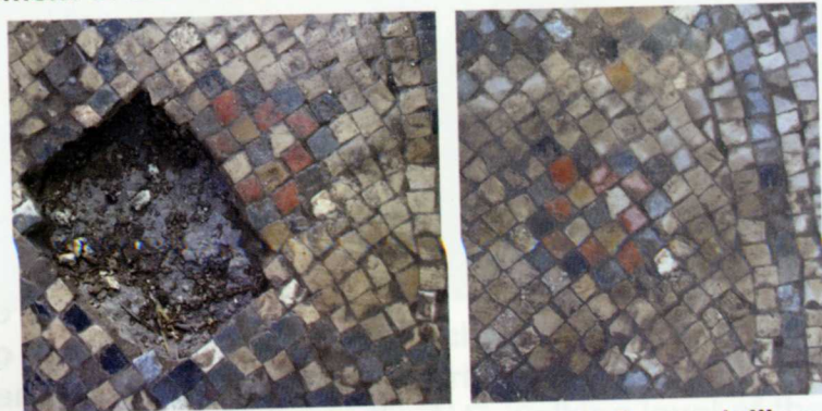
Fig. 86, Hippos, NWC, The northern annexe. A part of a medallion, situated in the central part of the room, was renovated.
